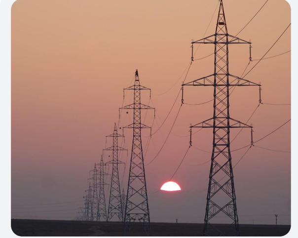
H.741 REF. 154 KV KARAMAN-EREĞLİ 102,8 KM ENERJİ İLETİM HATTI PROJESİ
